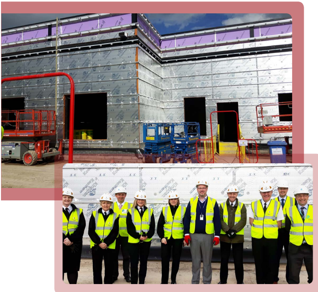
Visit to the new shared police and fire Operations Communications Centre, currently under construction at Hindlip
